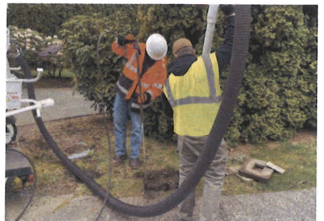
A two-person crew can excavate and vacuum debris from valve boxes for easy access
