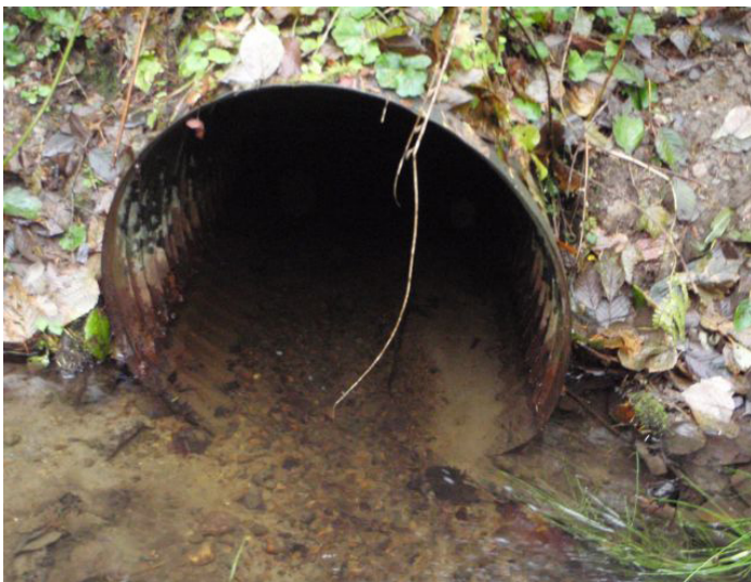
Figure 11. One old crossing (994125) was a 2.5 foot (0.76 m) round pipe which was a velocity barrier.
