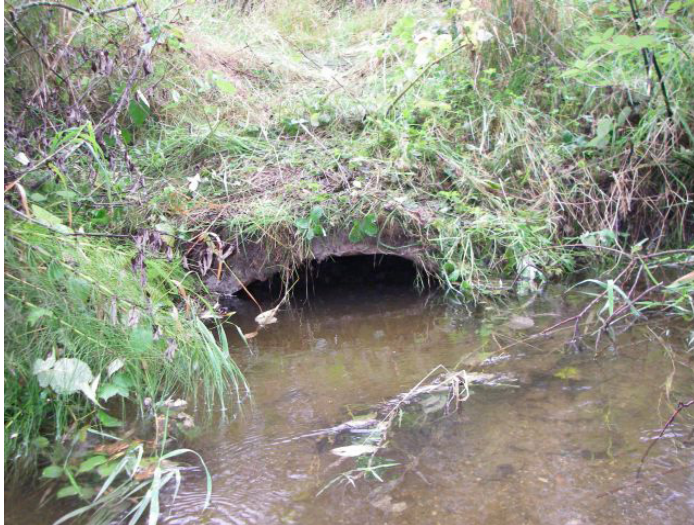
Figure 20. The old crossing was a 1 foot (0.3 m) round pipe that was a velocity barrier
