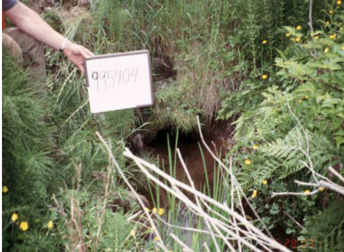
Figure 18. The old crossing was a 1 foot (0.3 m) round pipe that was a velocity barrier.
