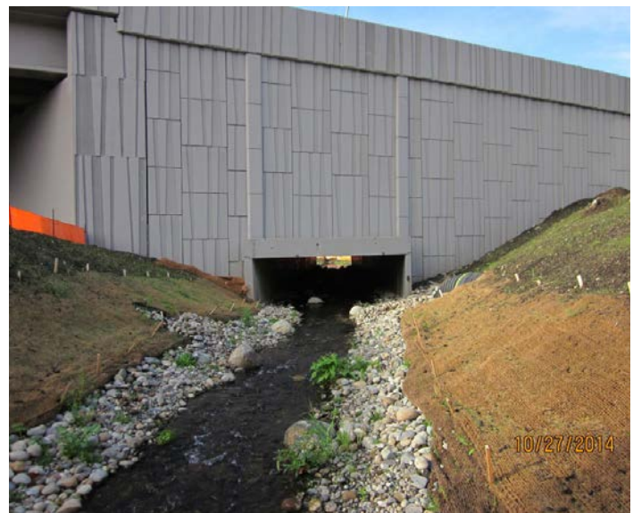
Figure 8. The new crossing is a 16 foot (4.88 m) wide culvert that provides 2.8 miles (4.57 km) of upstream habitat for sockeye and coho salmon, steelhead and resident trout.
