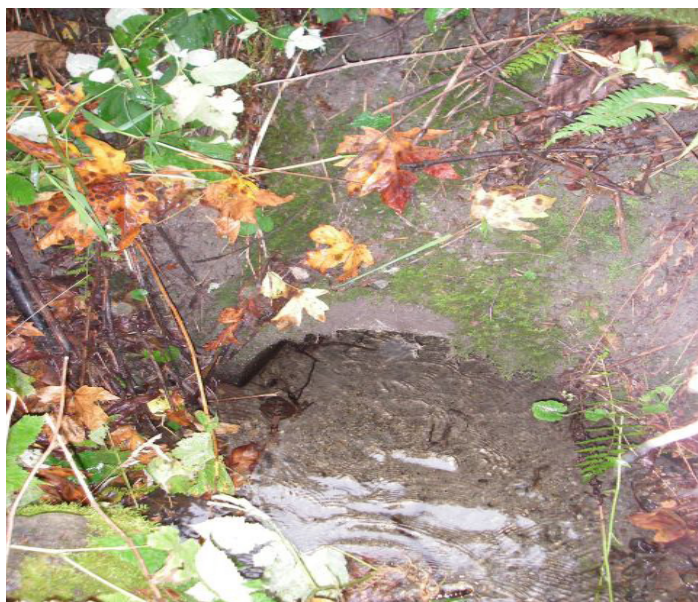
Figure 22. The old crossing was a 2 foot (0.61 m) round pipe that was a velocity barrier.
