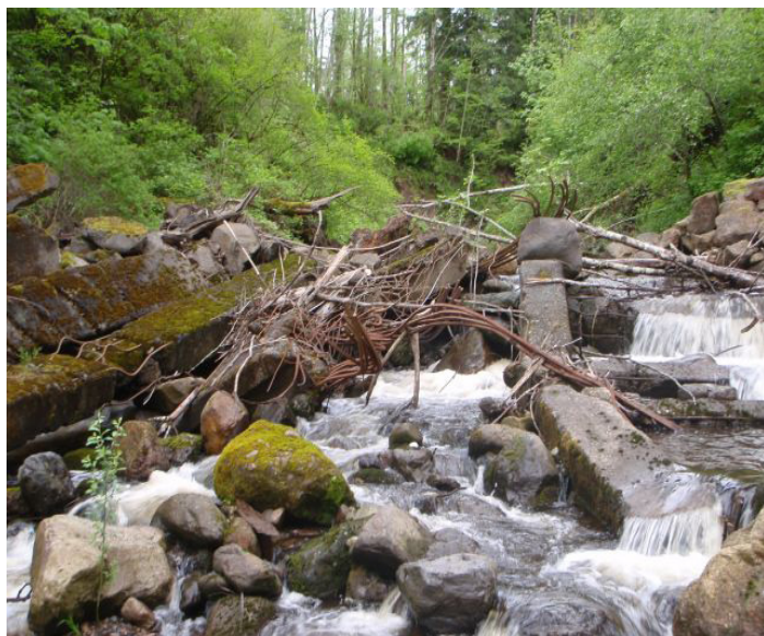
Figure 16. The stream underneath the Scatter Creek Bridge was filled with old bridge debris and was a barrier to fish passage.
