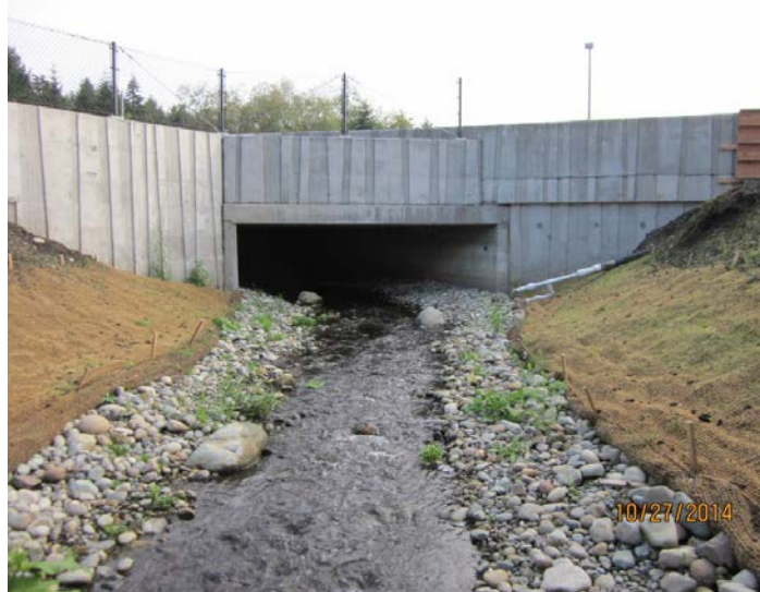
Figure 10. The new crossing is a 16 foot (4.87 m) wide culvert that provides 2.08 miles (3.35 km) of upstream habitat for sockeye and coho salmon, steelhead and resident trout.
