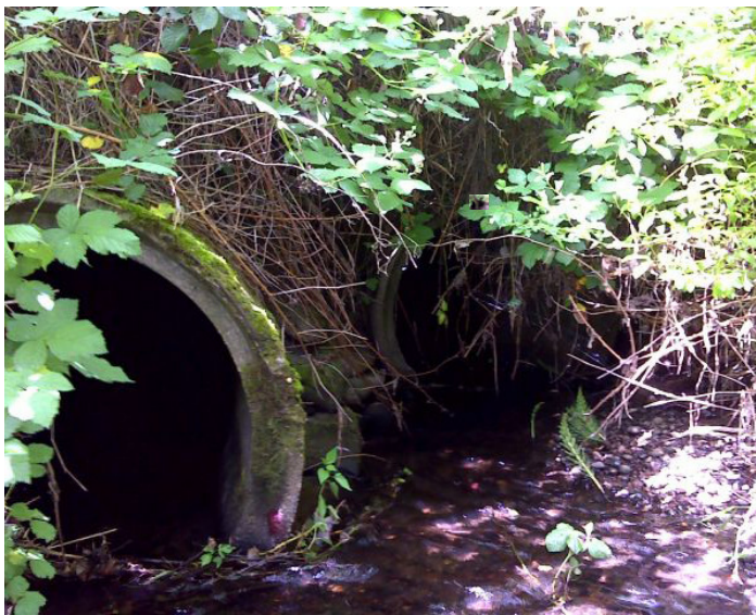
Figure 7. The old crossing consisted of twin 3 foot (0.91 m) round culverts that were velocity barriers.
