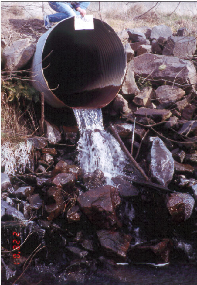
Figure 24. The old 4.5 ft (1.4 m) diameter corrugated metal culvert was installed when SR 504 was rebuilt following the 1980 Mt. Saint Helens eruption. The old crossing required repeated maintenance due to the geomorphic instability of the creek and road following the eruption. The crossing was a barrier to fish passage due to an excessive water surface drop at the outlet.
