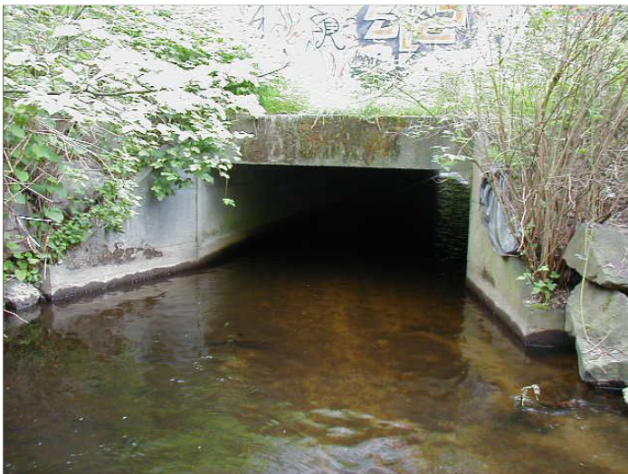
Figure 12. The old crossing was a 10 ft (3.0 m) wide by 6 ft (1.8 m) high box culvert that was undersized for the channel, resulting in a velocity barrier to migrating salmonids during high flows. Stream bed grade controls installed throughout the downstream reach to minimize channel regrade and facilitate fish passage were underperforming and some were deteriorating. Serious flooding in 2007 along the Little Bear Creek corridor prompted planning to improve hydraulic capacity of the SR 202 crossing.
