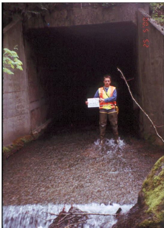
Figure 28. The old crossing was a 10 ft (3.0 m) by 10 ft (3.0 m) concrete box culvert that was a barrier to fish passage due to an excessive water surface drop at the outlet and sheet flow through the culvert.
