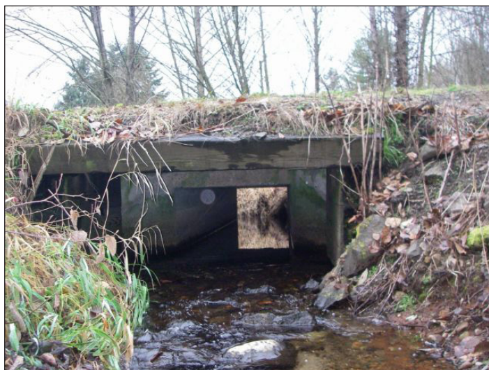
Figure 14. The old crossing was a box culvert 4 ft (1.2 m) wide by 3 ft (0.9 m) high and was a partial barrier to fish passage due to excessive velocity at high flows. The culvert was retrofitted during past highway work but did not adequately provide fish passage long term.
