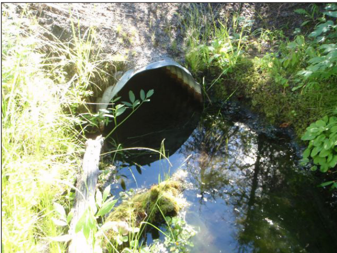
Figure 34. The old crossing was a 2 ft (0.6 m) diameter corrugated metal culvert with a surface grate at the inlet that was a barrier to migrating steelhead as well as bull trout and resident trout.
