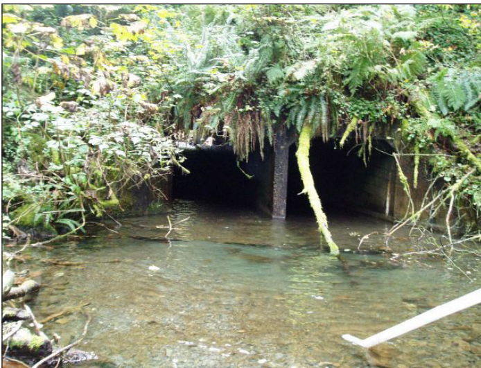
Figure 4. The old crossing was a double barrel concrete culvert that was a barrier to fish passage due to excessive velocity through the structure.
